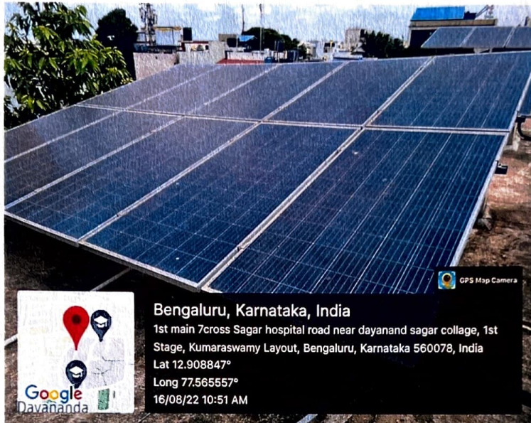
SOLAR ENERGY PANELS ON BUILDING ROOFTOP
